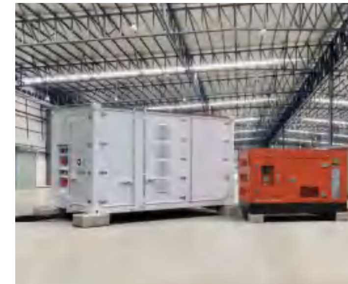
Power Bank & DG
