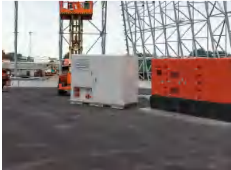
Lifter Rated power: 3*11kW Peak Power: 60kW Operation: 10h/day
