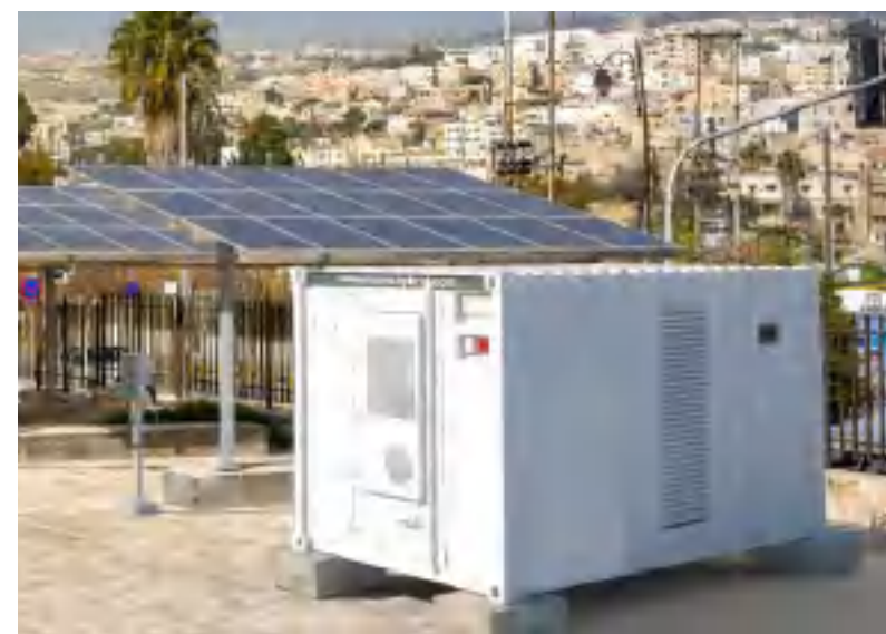
EV Charging Solar + BESS
