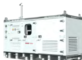
Battery & Diesel/Gas Genset
